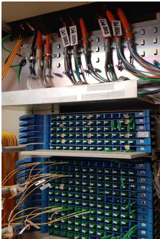
Mumbai Fibre Cables
