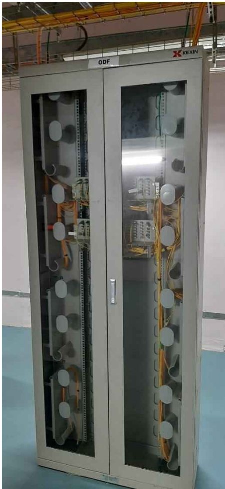
Bengaluru Fibre Cables
